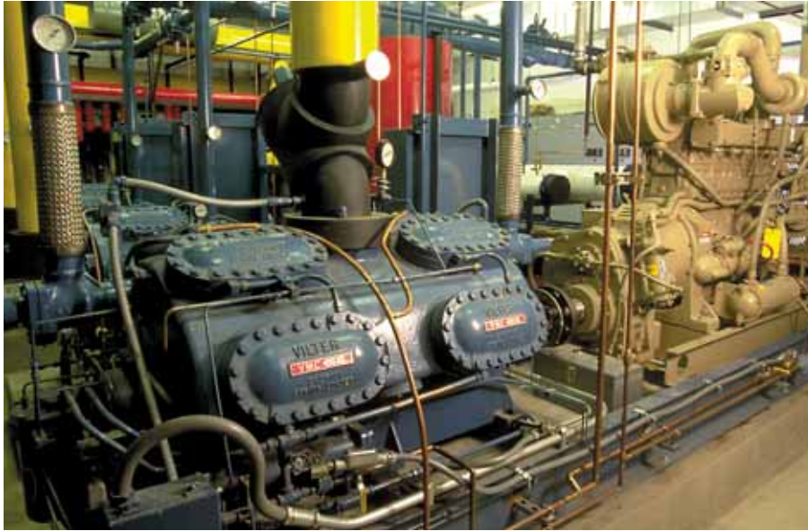
A 350-horsepower Cummins natural gas engine-driven chiller with 160-ton Vilter compressor are key components of a hybrid ice-making system at the Super Rink.
